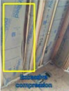
Grade II: Not Compliant
