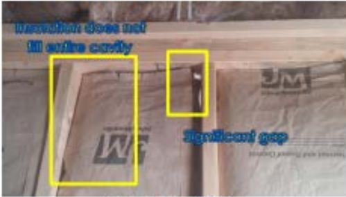
Grade III: Not Compliant
