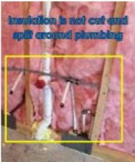
Grade III: Not Compliant
