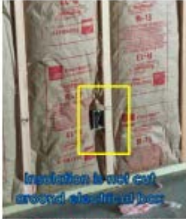
Grade II: Not Compliant
